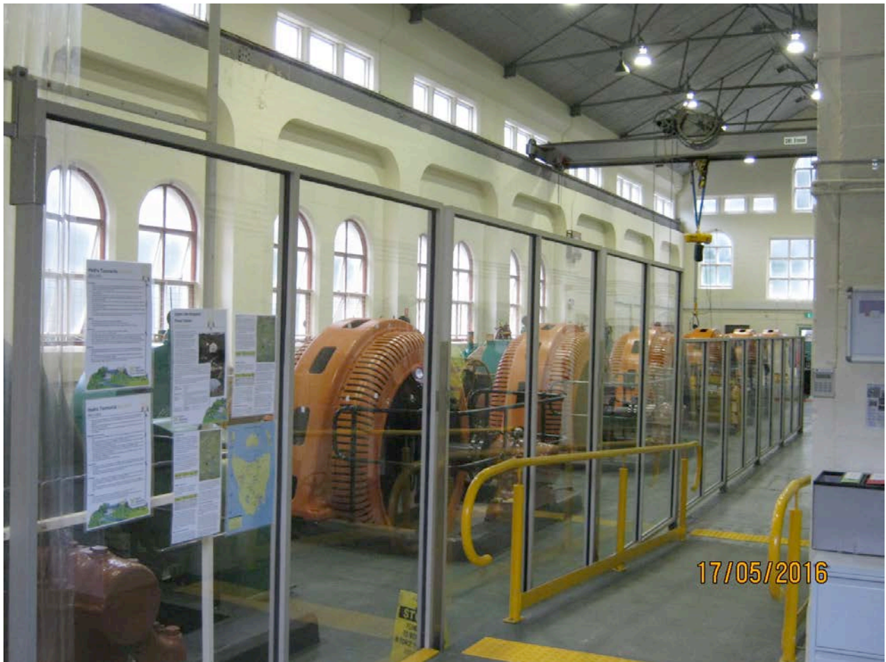
Bank of Turbines. This was good old English engineering these turbines have had little maintenance since they were installed 102 years ago. How they got them there was a feat in itself. There were no formed roads in this part of Tasmania at the time they were installed. Even the building has an architectural quality about it.
